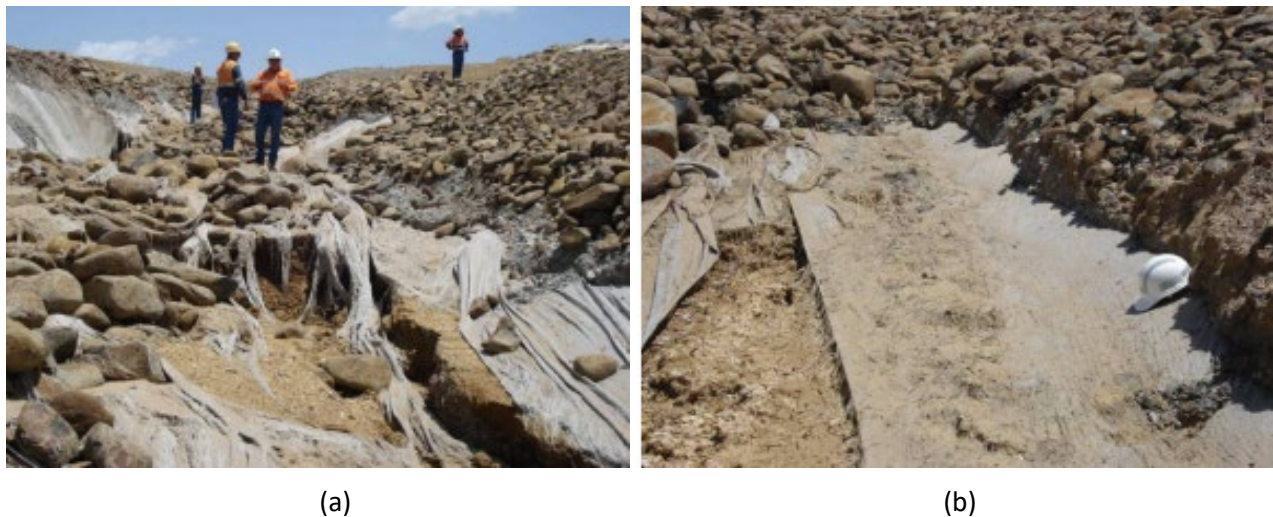
Figure 11 (a) Erosion failure of a rock lined drain; (b) Detail of the scour (hardhat shows rock scale)
