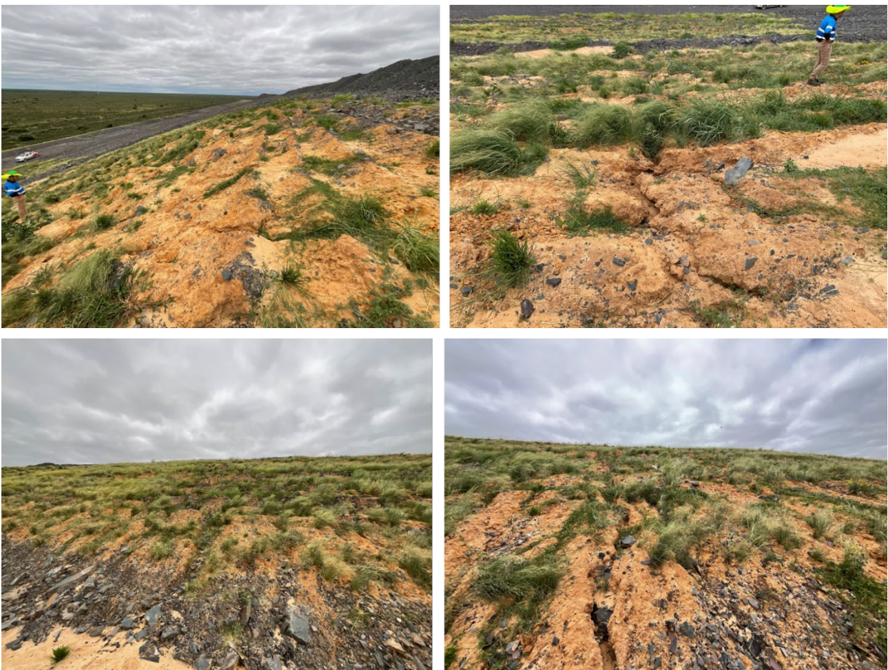
Figure 7 Trials assurance findings – side slope erosion
