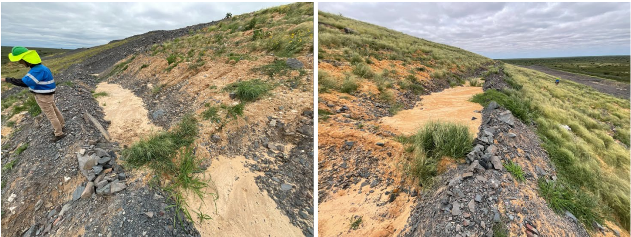
Figure 8 Trials assurance findings – siltation of stormwater structures
