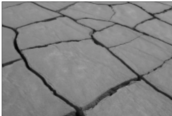
Figure 3: Desiccation cracks on surface.
