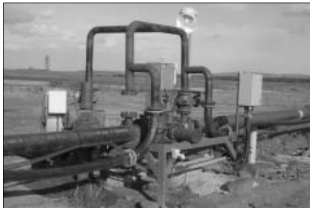
Figure 9: Hydraulic pinch valves and flushing system.
