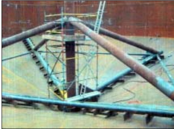
Figure 20: Comalco Alumina Refinery – 22 m Paste Thickener (2004).
