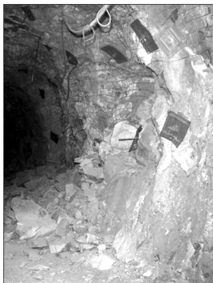
FIG. 18 Rockburst in 33N1 (porphyry), moderately controlled by support system - prior to wall meshing becoming standard in porphyry
