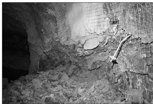
FIG. 1 Development wall burst triggered by a Nutli Magnitude 2.1 event locating 40 m away. Most of the damage was below the wall support line, but a rebar can be seen dangling. The brittle rock “shattered” out around the bar, never soliciting its’ full strength
