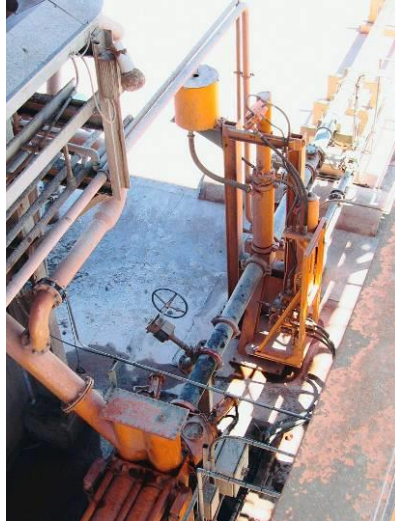
Figure 20 Seat valve pump at Plutonic Gold Mine with high pressure dampener
