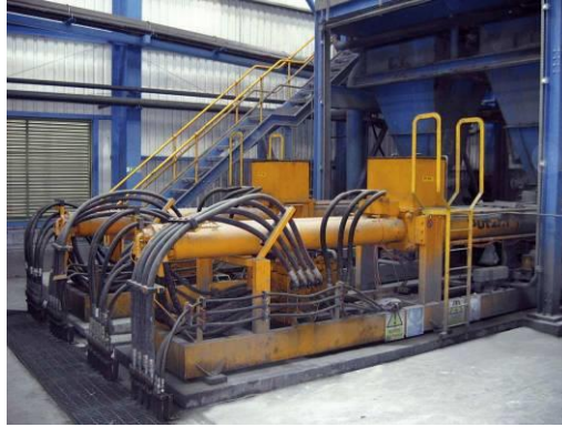
Figure 24 HSP 25.100 double piston pump with PCF at Lisheen Mine, Ireland
