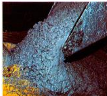
Figure 6 Stiff plastic concrete mix with a maximum grain size of 32 mm for backfilling
