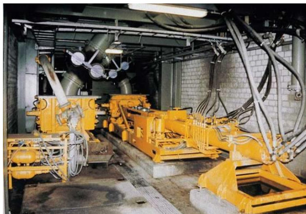
Figure 14 Paste pumping station at Walsum Coal Mine
