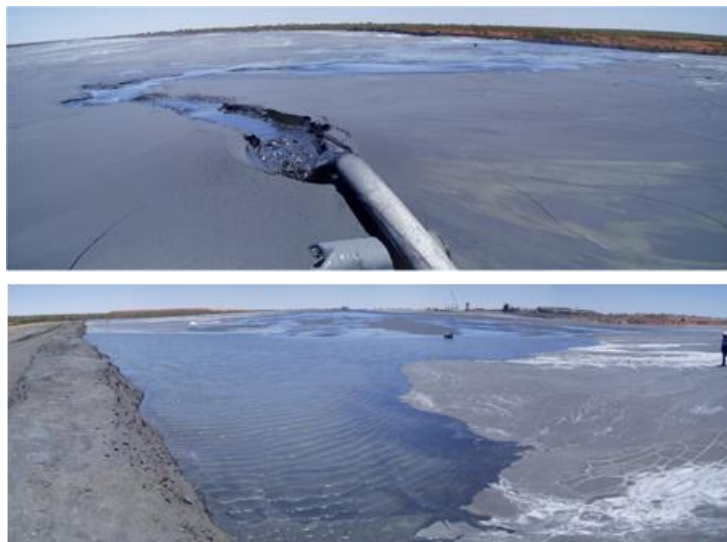
Figure 8 Ponding against the toe wall at the intersection of two advancing cones
