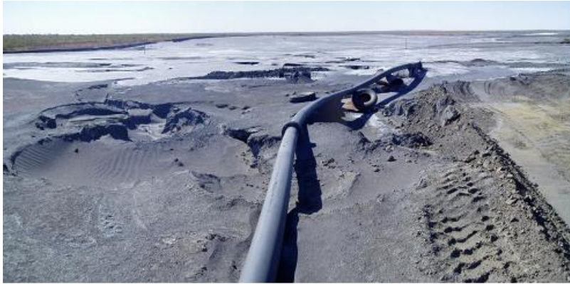
Figure 9 Typical delivery point showing HDPE pipe issues
