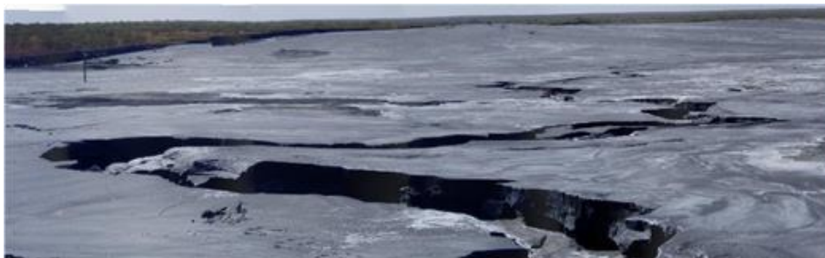
Figure 10 Typical flushing scour at Osborne
