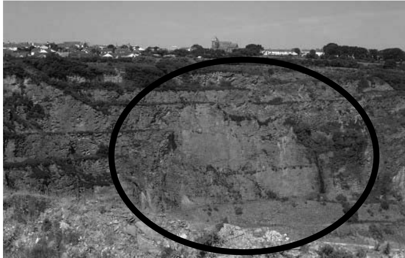
Figure 2 Current profile of the West face, Delabole Slate quarry taken from the haul road at the crest of the East face looking west with the 1967 failure highlighted
