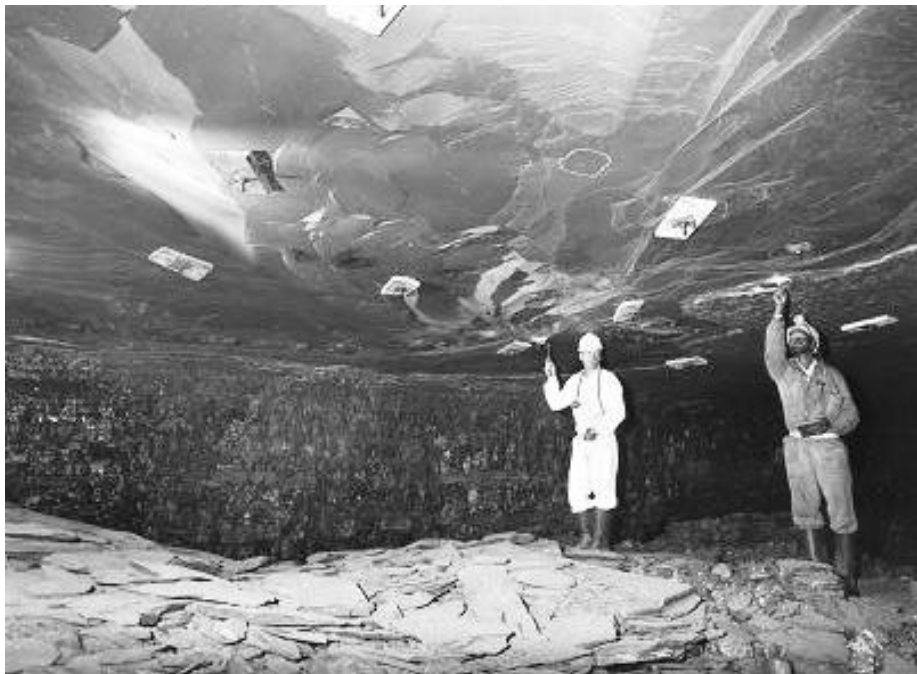
Figure 12 General view of the roof failure
