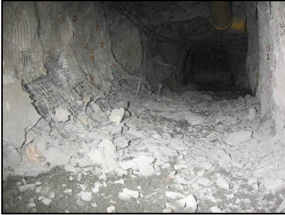
Figure 4 Damage in haulage drift EP-224-47E following the January 11th 2007 event (lower part of North wall ejected)
