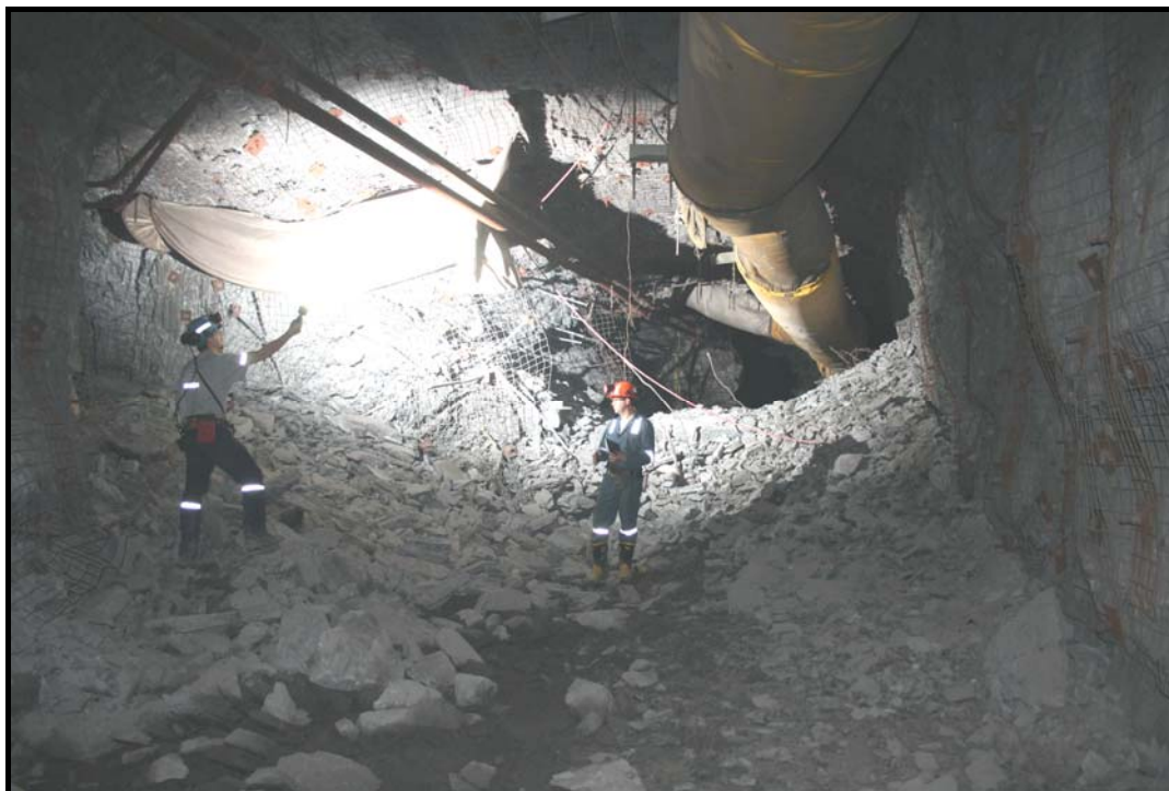
Figure 3 Damage in haulage drift EP-164-20W following the April 1st event (south pillar ejected)
