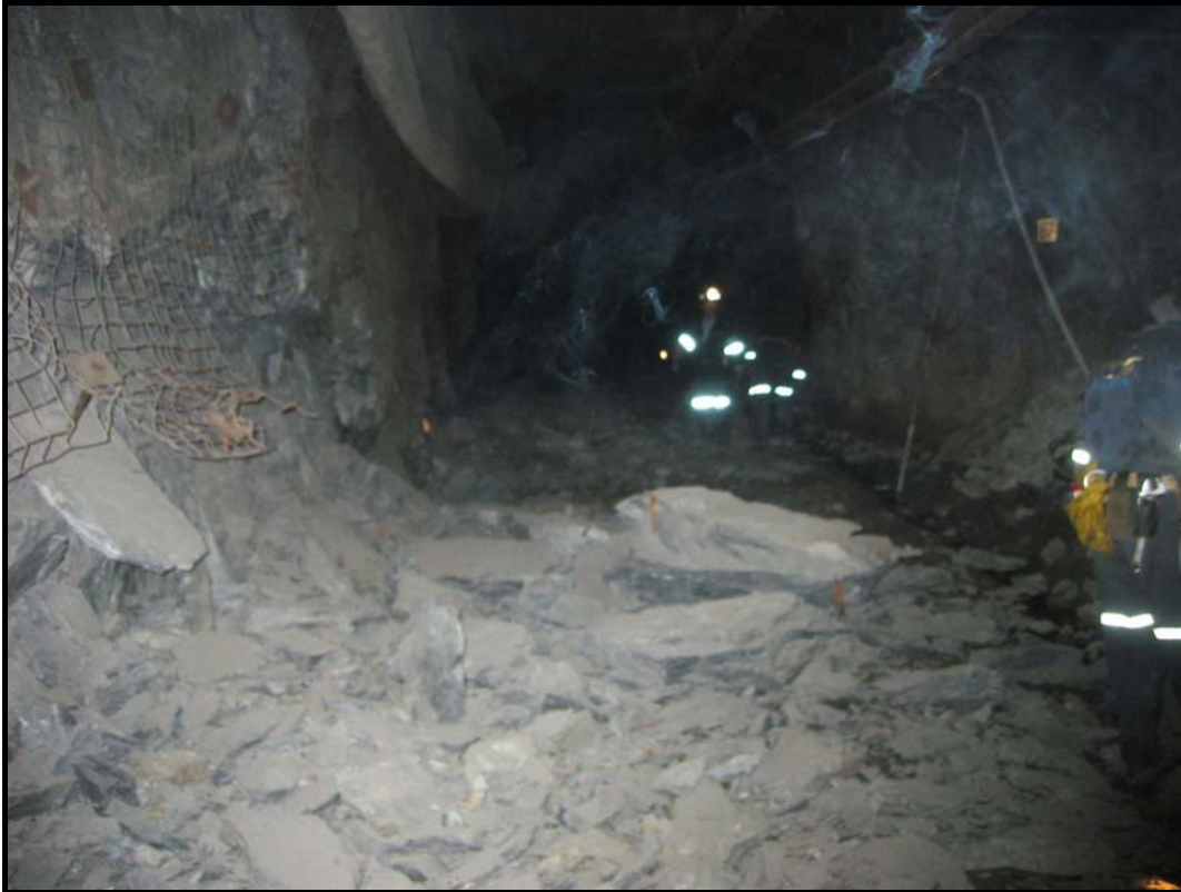
Figure 2 Ejected material in 149-20W haulage drift following the November 27th 2002 event (lower part of North wall ejected)
