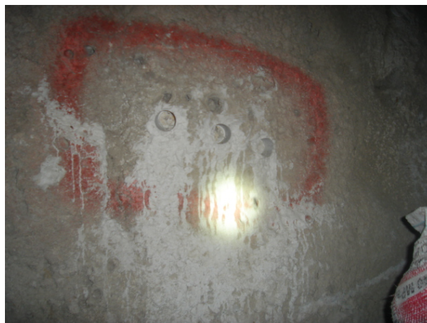
Figure 4 Photo showing the cores drilled out of the sidewall at grade elevation
