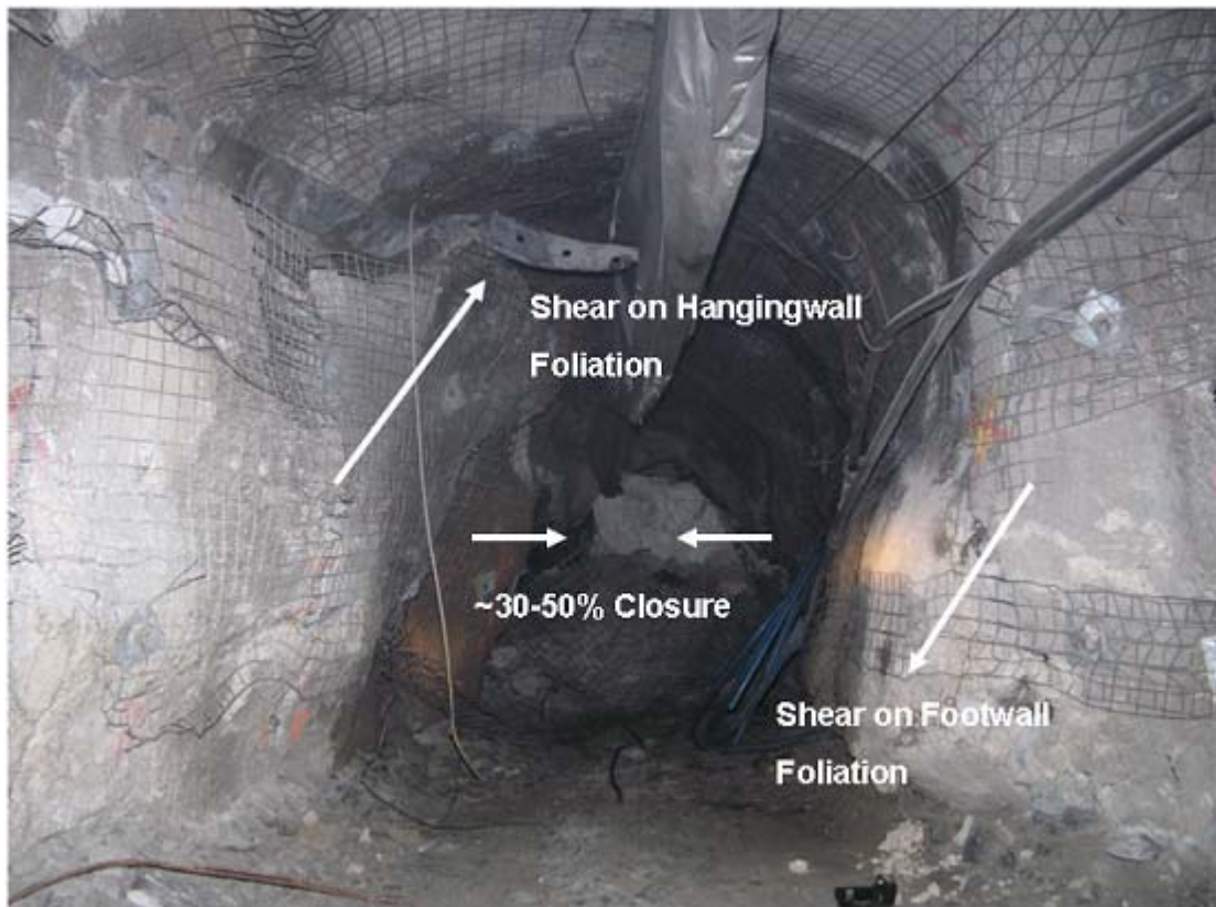
Figure 11 Drive exhibiting advanced stage of wall deformation. Serviceability has been lost
