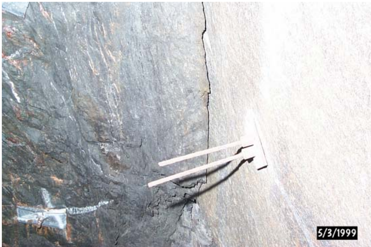
Figure 7 Initial indication of high deformation – dilation/shear of the hangingwall/back contact
