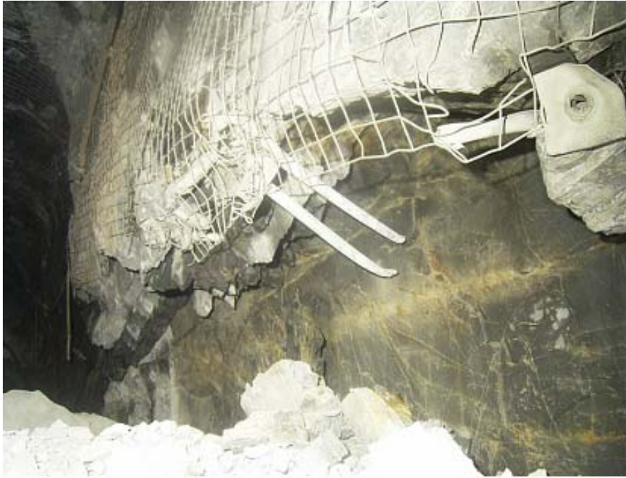
Figure 5 Guillotining of friction bolts installed in the footwall. Note the sense of shear indicated by the damage to the bolts
