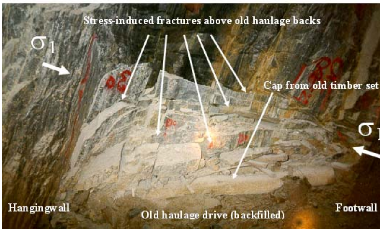
Figure 1 Stress-induced fracturing above the backs of 1950s haulage drives at Big Bell
