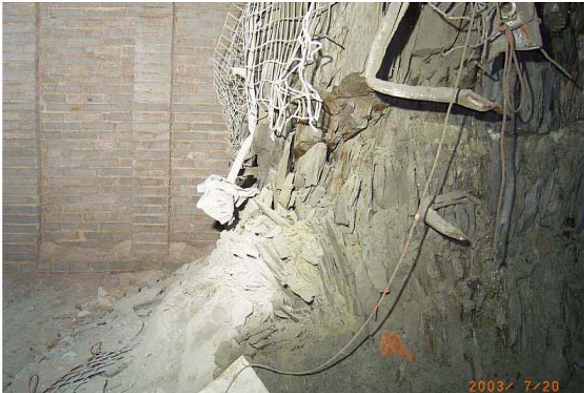
Figure 8 Buckling of the lower footwall
