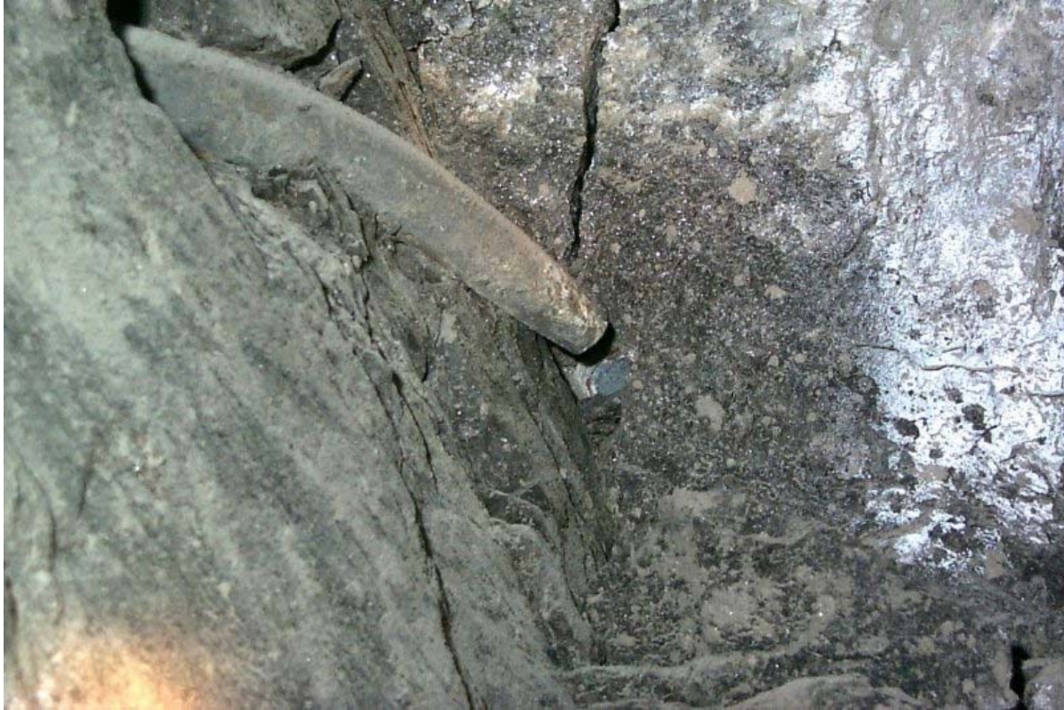
Figure 6 Necking and guillotining of friction bolts installed in the hangingwall. Note the sense of shear indicated by the damage to the bolts
