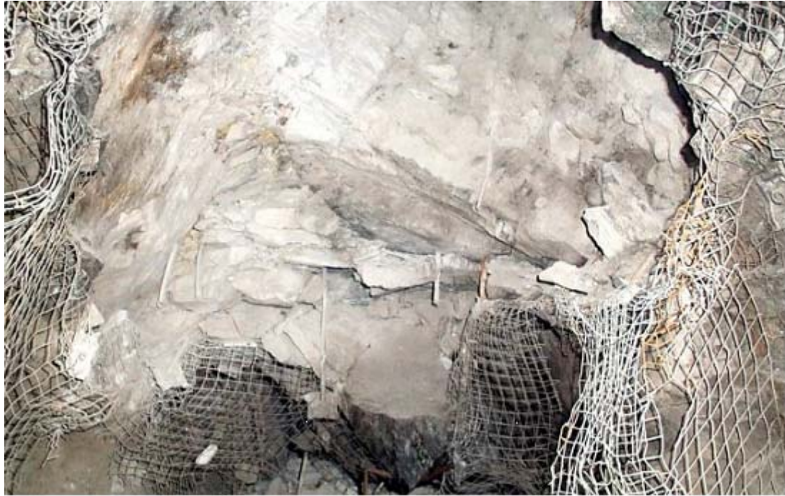
Figure 10 Stress-induced fracturing above the backs of an ore drive at the Yilgarn Star gold mine
