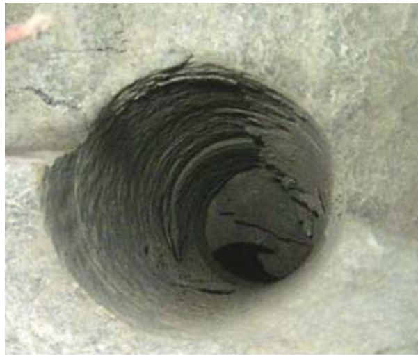
Figure 4 Shearing of 89 mm diameter sludge sampling holes in ore-drive hangingwall
