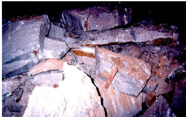
Figure 13 Roof and support system failure caused by dynamic loading
