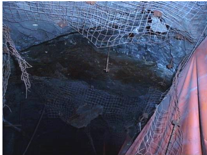
Figure 2 Roof failure in access drift, caused by mining in the upper levels
