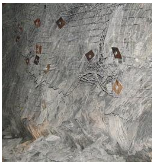
Figure 1 Squeezing ground failure in the lower section of a drive due to the support system not extending to the floor
