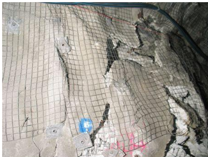
Figure 3 Mesh applied over in-cycle FRS is a common practice in Australia where the ground conditions are poor
