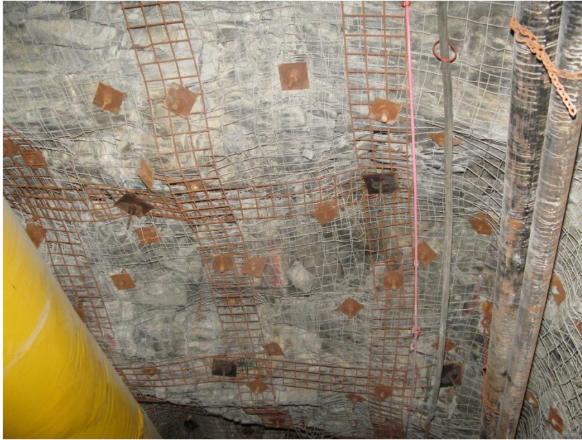
Figure 4 Mesh straps installed where the sheets of mesh overlap is a common practice in Canada where the ground conditions are poor
