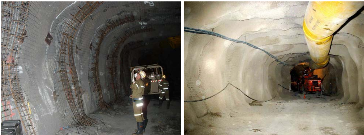
Figure 8 Reinforced shotcrete arches at Perseverance Mine in construction (left) and completed (right)
