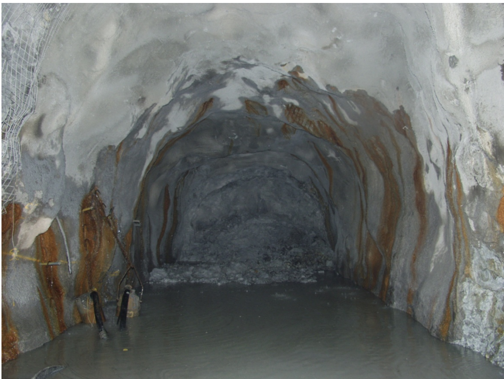
Figure 3 815 level access at Favona — showing exceptionally poor ground conditions at the excavation face following intersection with the Main Fault. Large accumulation of water with two 37 kW pumps for dewatering
