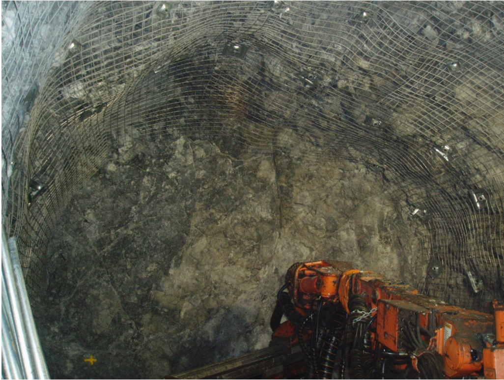
Figure 2 Decline excavation face during the ground support installation phase showing good ground conditions
